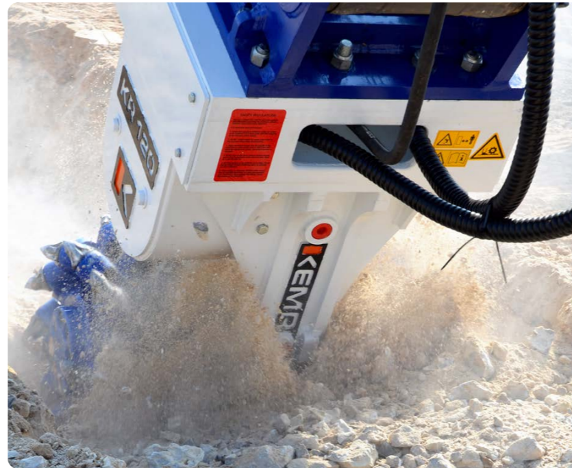
▲ A KR 120 in operation.
